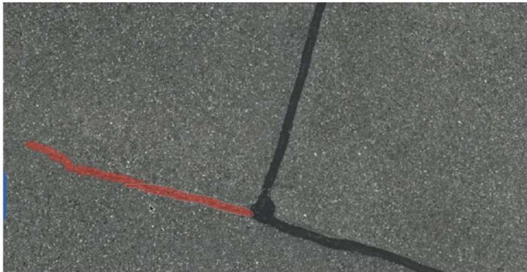
Figure 6: A close-up view of a crack at the Dubendorf Airbase that was previously repaired but has since continued to expand.
