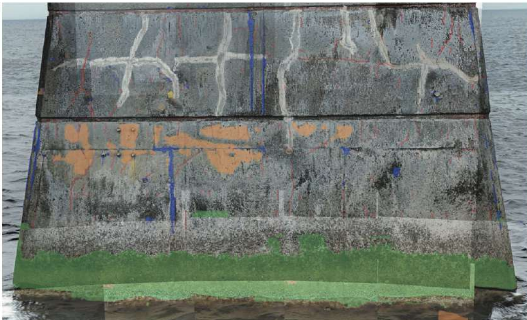
Figure 3: High-resolution analysis of the Storebælt Pillar 3, south face, bottom region, performed by IBM Inspecto. This view consists of 30 high-resolution images seamlessly stitched together by our algorithm. Our finely-tuned AI foundation model identifies various defects: cracks (red), net-cracks (orange), spalling (blue), rust (yellow), cracks with precipitation (pink), and algae (green).
