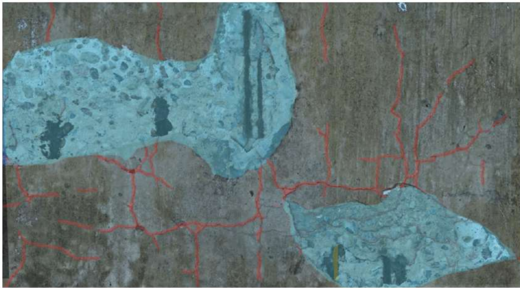
Figure 5: IBM Inspecto results on the Stenungsund Bridge: the image highlights significant instances of spalling with corroded rebars, accurately detected by our model.
